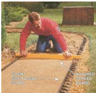
SMOOTH AND LEVEL the sand using a notched screed board riding along the edging for a guide. Include a slight tilt for good drainage.
