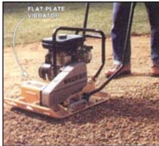
5. TAMP THE SUBBASE using a flat-plate vibrator (rented at $40 a day). Work in a circular motion and compact the area twice.
