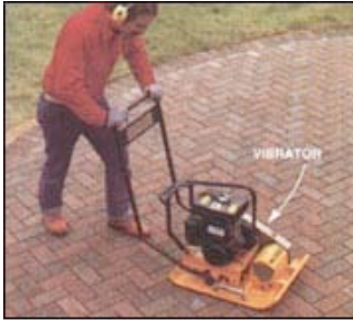
14. TAMP THE PATIO with a flat-plate vibrator after the pavers are installed. Tamp entire outside edge first, then circle in.
