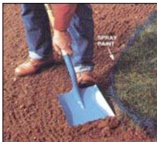
2. REMOVE SOD in an area extending 8 inches beyond the boundaries of the patio. Spray paint indicates the excavation line.
