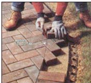
11. MARK PAVERS that run "wild" into the border area. Then remove the paver, cut to size and place back in position along with border paver.
