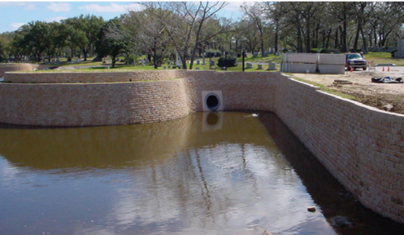
Outlet pipes were designed so the batter was the same as the wall.
