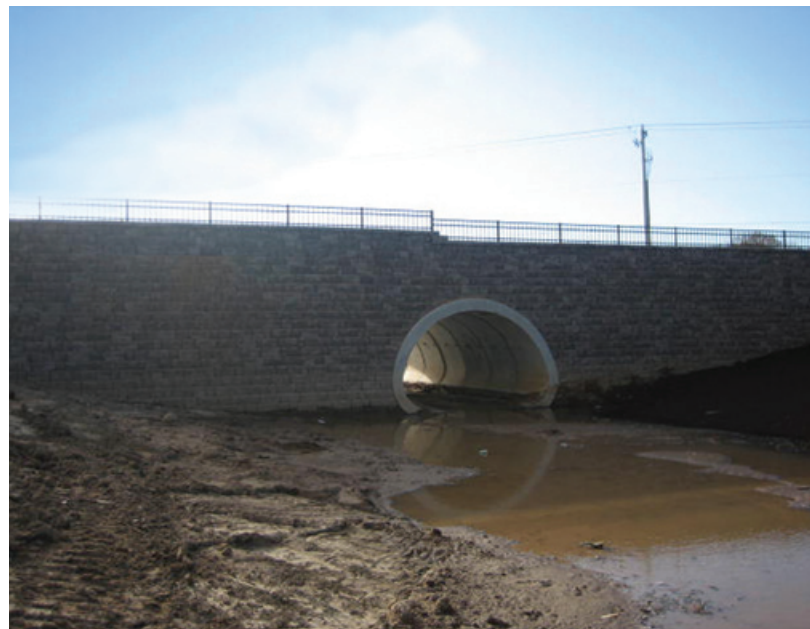
The contractors needed to build the detention pond quickly, before it filled with storm water.
